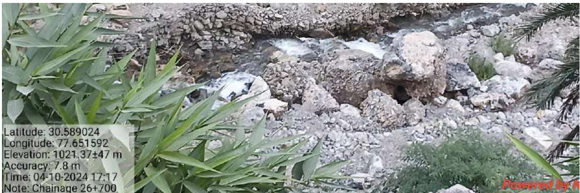
Location RD 25+500 to 26+700 Gabion wall constructed: nallah not obstructed and water channelised
